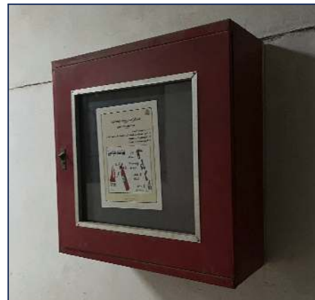
Figure (44): Fire extinguishers in workspace
